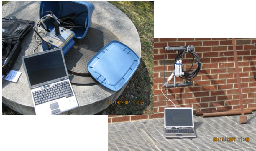
Figure 2 - Flow Monitoring and Wet Well Level Data Loggers
