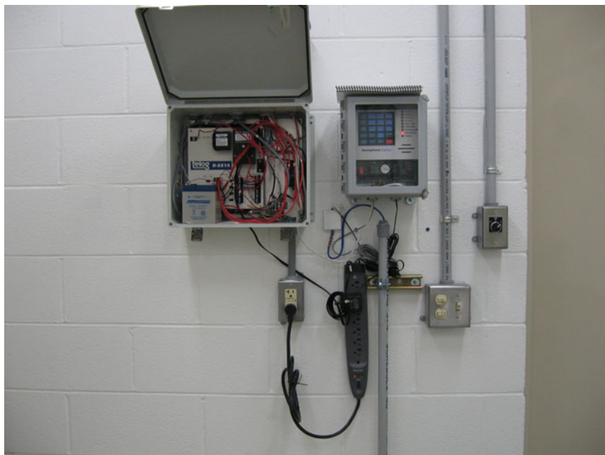
Figure 11 – Photograph of Installed 14 Channel Data Logger (left)
