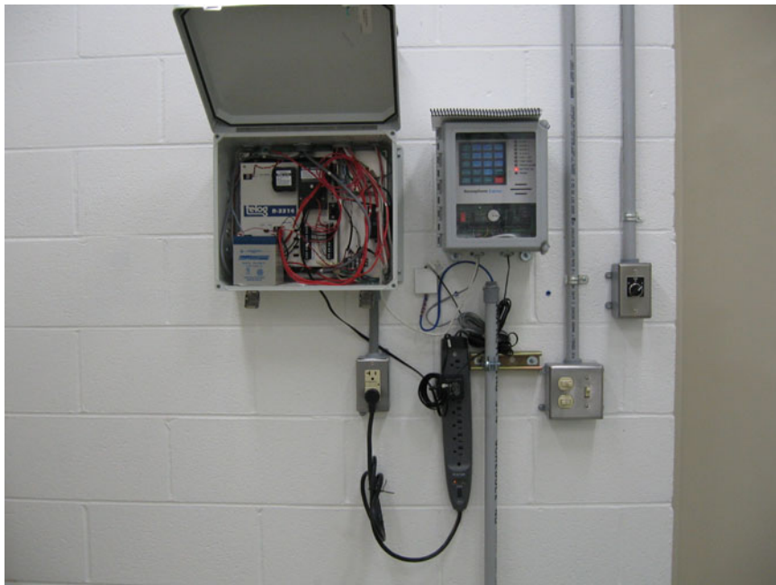
Figure 11 – Photograph of Installed 14 Channel Data Logger (left)
