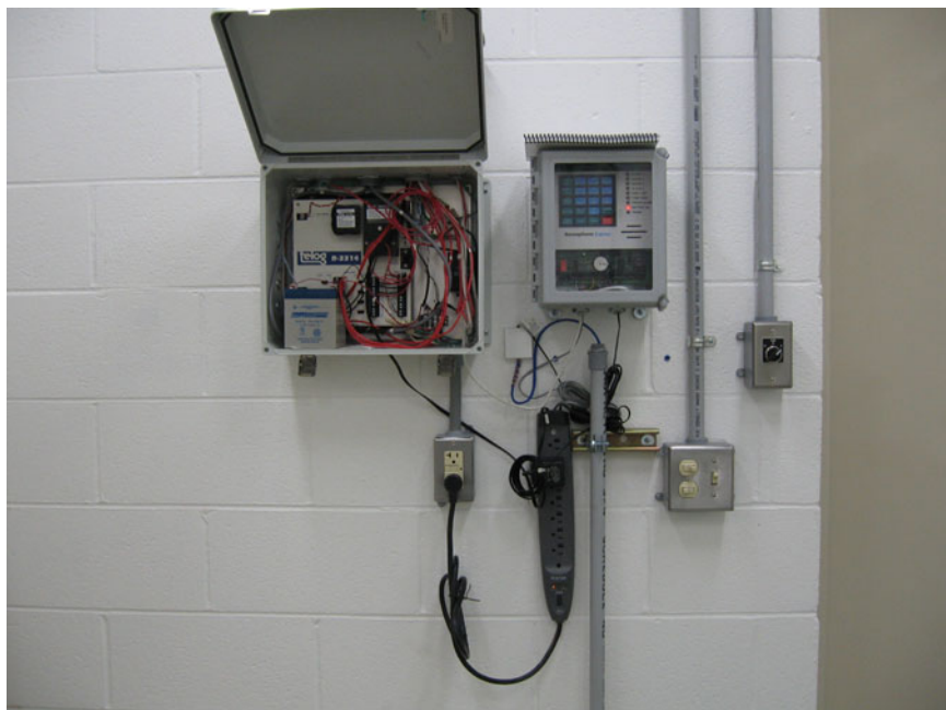
Figure 11 – Photograph of Installed 14 Channel Data Logger (left)
