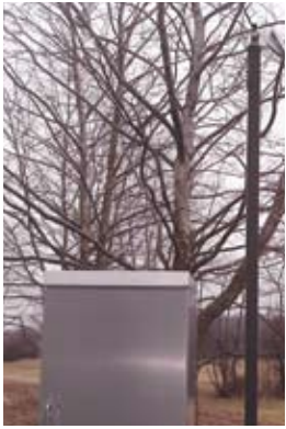
The Telog RTUs used for this project were provided with solar power, eliminating the need for AC power or field visits to change batteries.
