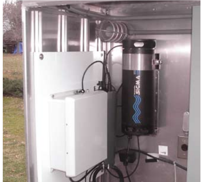
The RTUs employ switched packet protocol, which uses the Ethernet capabilities of the existing cellular infrastructure to push data in 15-minute intervals to the remote server.
