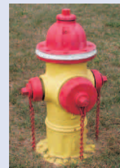
This hydrant flowed less than 500 gpm, therefore, its caps and bonnet are painted RED .
