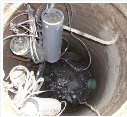
Sigma flow monitors and Telog recording telemetry units during study.
